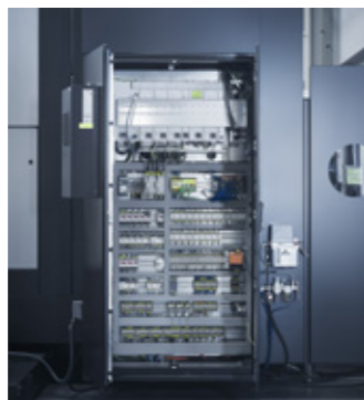
Climatised electrical cabinet.
